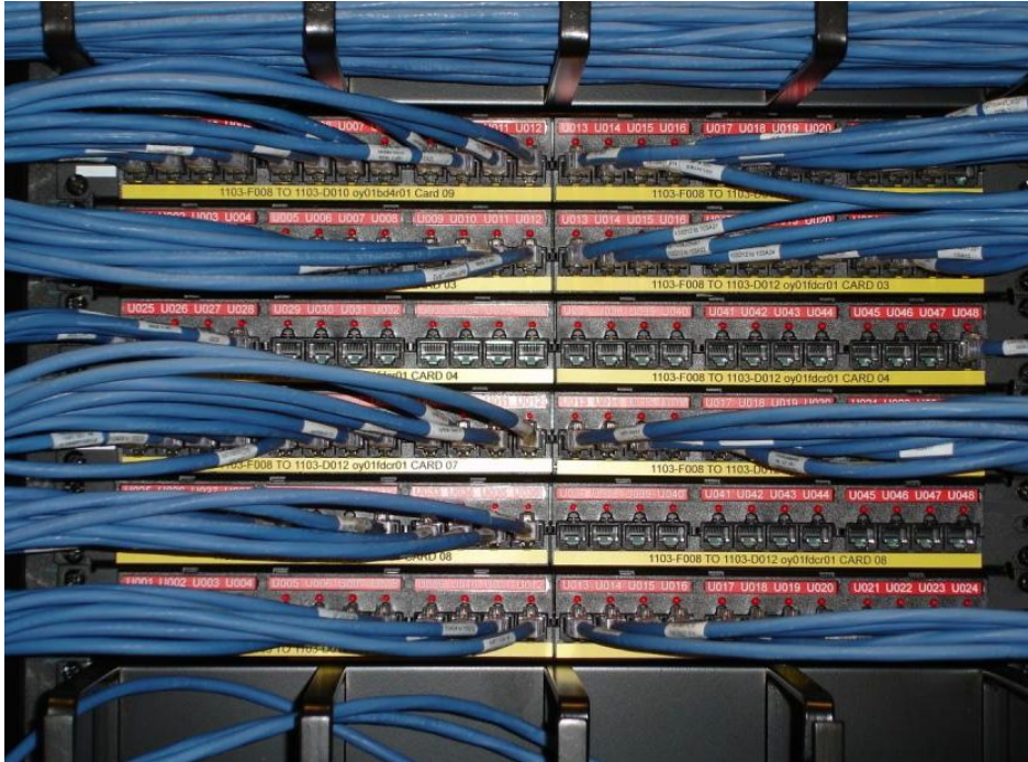
Figure 14-16 Example of Labeled Termination Ports and Equipment Cords
