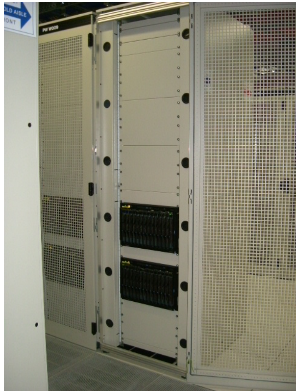
Figure 14-12 Blanking Panels Installed in Empty RUs
