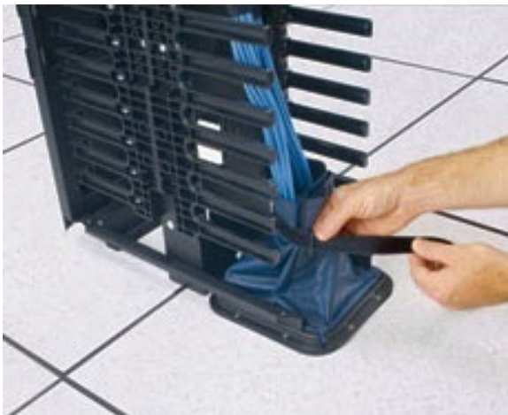
Figure 14-19 Gasket Seals Off Access Floor Tile Cutout In Vertical Cable Manager
